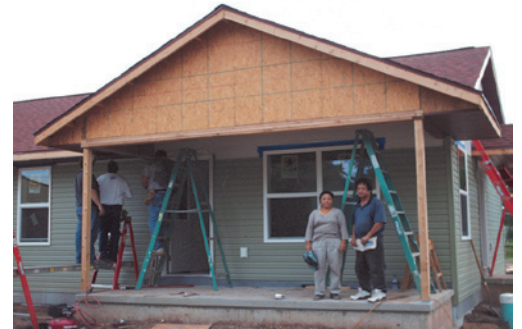
Kao Yang and Yia Thao stand on their front porch during construction of their home at 459 S. Military Road, FDL. Many thanks to our corporate sponsors for their funding efforts: Lowe's, FDL Area Foundation, Wells Fargo, Grande Cheese, Alliant, First Weber, MidStates Aluminum.
